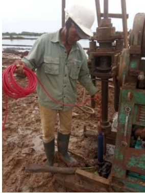
Gambar 2.28 Vibrating Wire Piezometer
