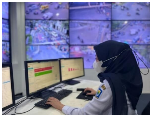
Gambar 2.2 Central Control System Room ATCS
