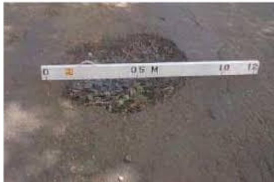
Gambar 2.13 Lubang ( pothhole ) Sumber : Bina marga no.03/MN/B/1983
