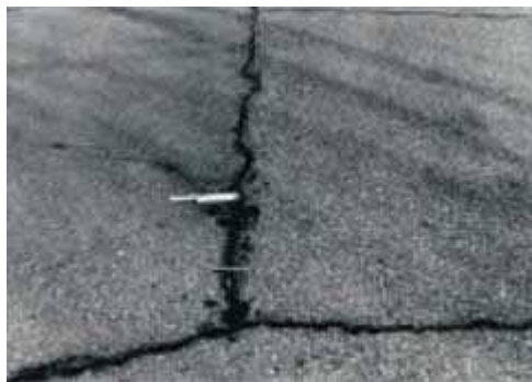
Gambar 2.8 Retak Sambung ( Joint Reflec Cracking )
