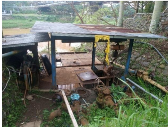
Gambar 2.9 Bangunan Intake IPA Purwaharja PDAM Tirta Anom
