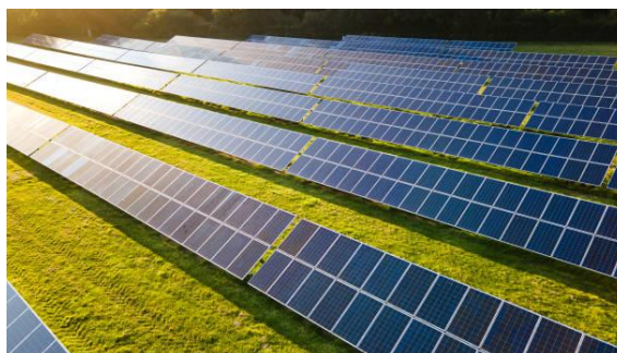
Gambar 2.5 PLTS Ground-mounted (ESDM, 2019)
