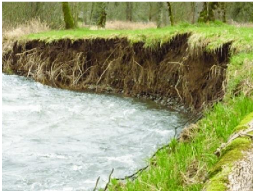
Gambar 2.11 Erosi Tebing Sungai ( River Bank Erosion )
