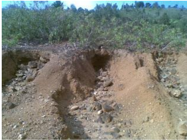
Gambar 2.12 Erosi Internal ( Internal Or Subsurface Erosion )
