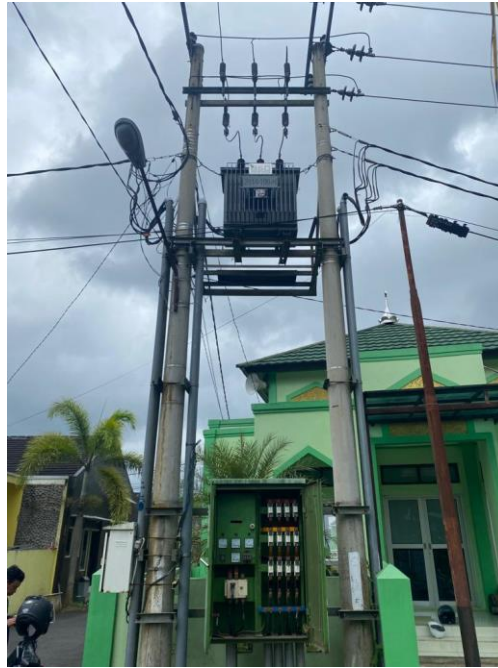
Gambar 3. 4 Transformator Distribusi PGGC
