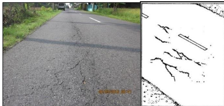
Gambar 2.8 Retak Halus ( Hair Crack )
