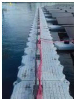
Gambar 2. 16 Marine grade DC cable (ESDM, 2021)
