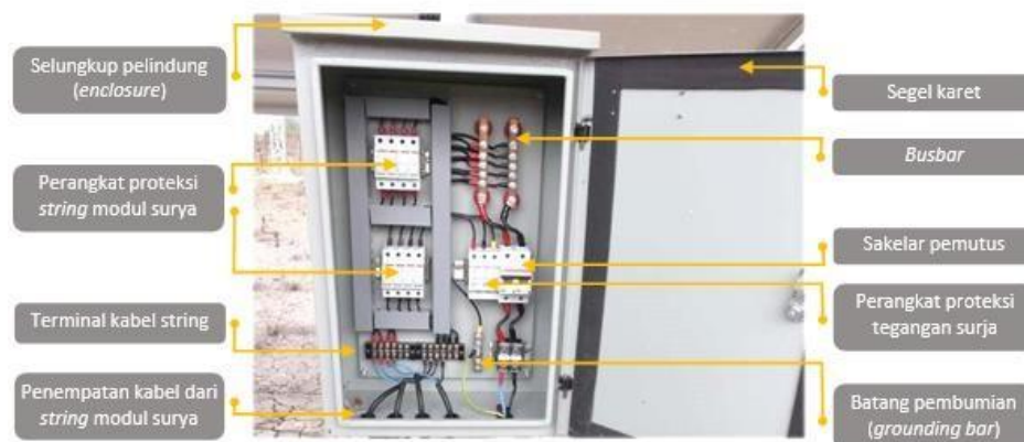
Gambar 2. 17 Combiner Box (sunwind,2022)
